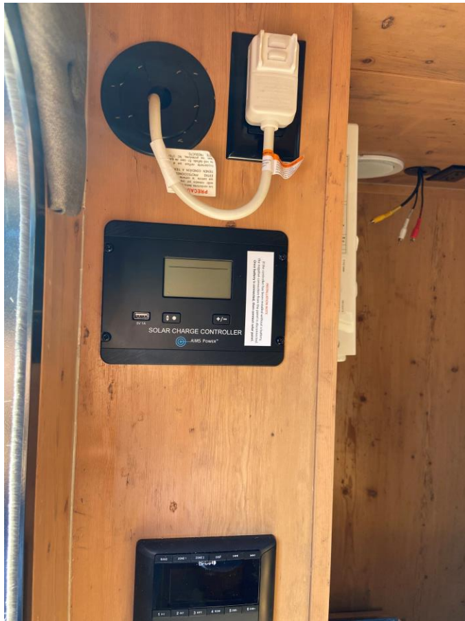
Solar Controller Location
