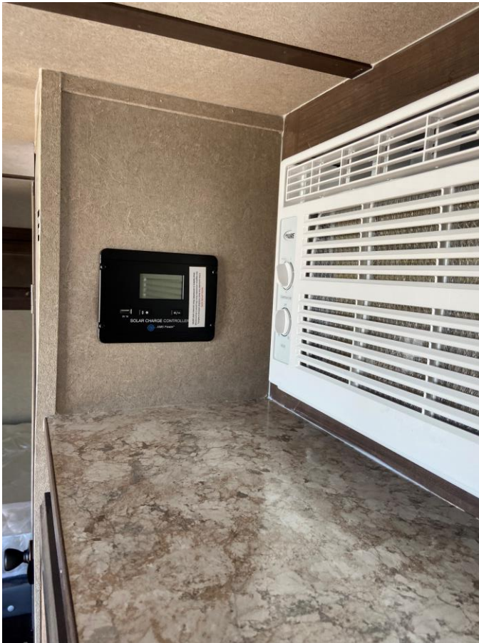
Solar Controller Location
